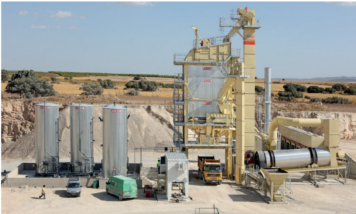
280 t/h asphalt plant (Spain). With InNOVA-G mixing tower. Equipped with 160 t capacity hot bins. Bitumen and fuel tanks electrically heated. 4.500 kg mixer. Equipped with cold process recycling system unloading in the mixer.
