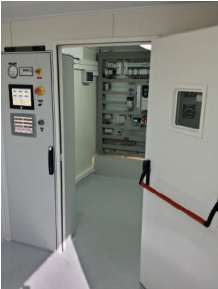
Electric panel in technical room.
