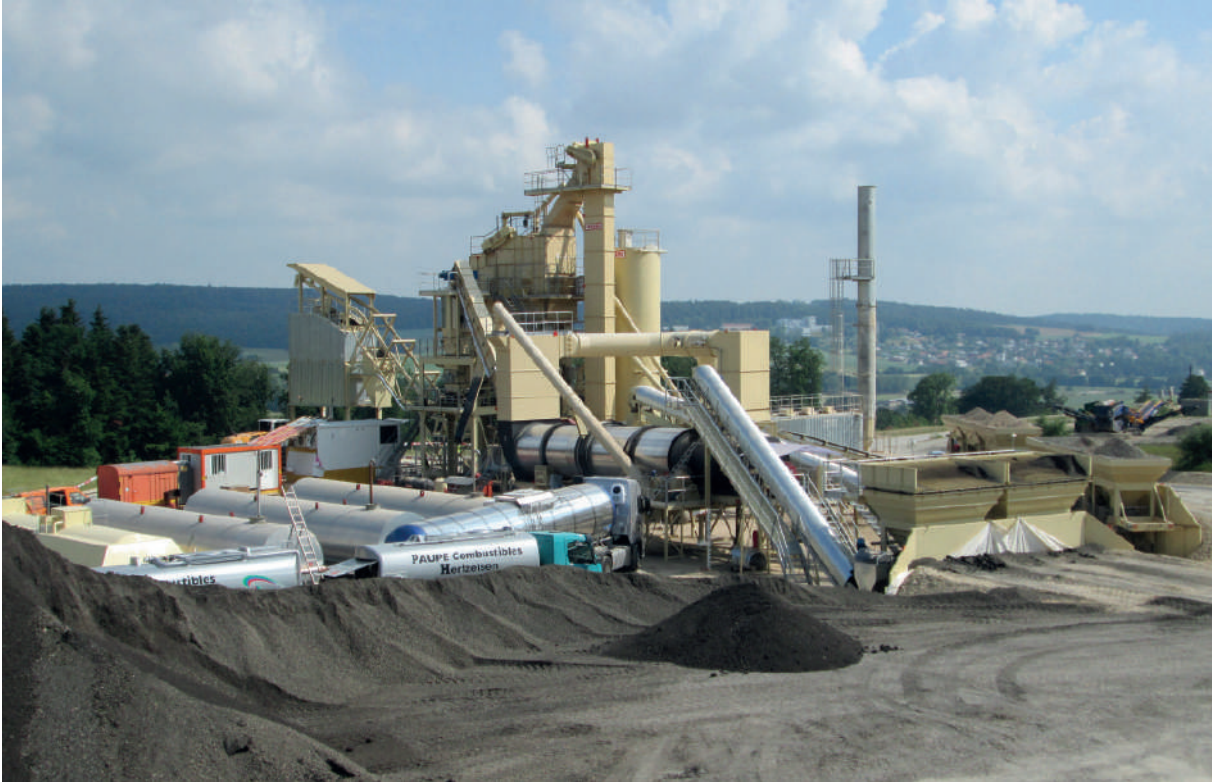
Hot process recycling equipment RC-120 installed in a M-280 asphalt plant (Switzerland).
