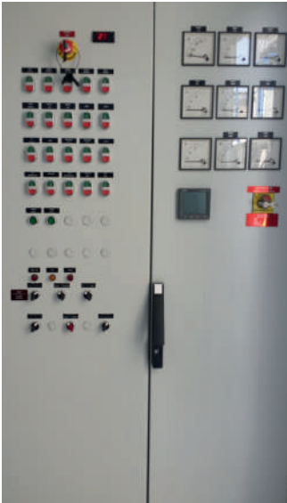
Electric panel in cabinets.
