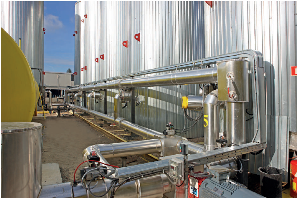
Electrically heated pipes in InNOVA 320 plant (Poland).
