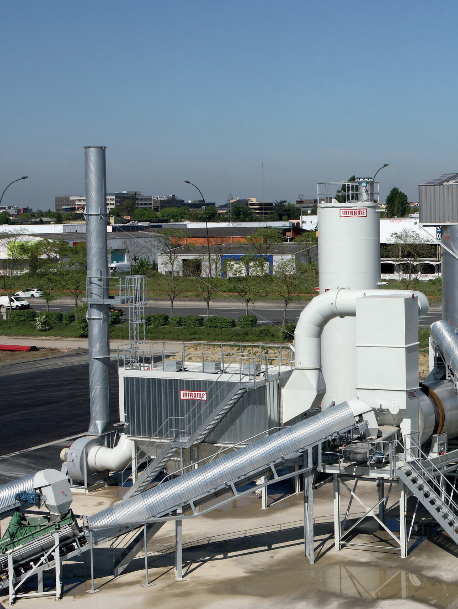
Flow-Mix 220 asphalt plant in France
