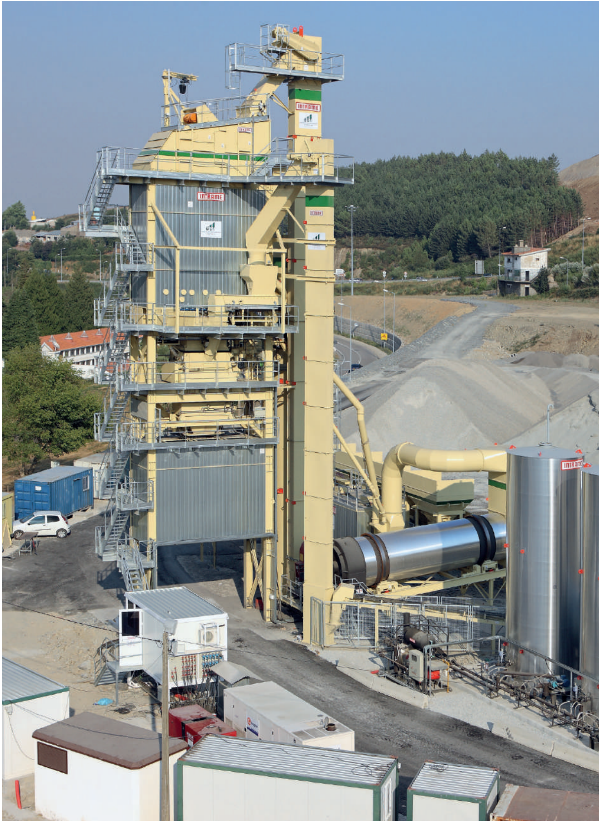
200 t/h asphalt plant (Portugal). With InNOVA-S mixing tower. Equipped with 90 t capacity hot bins and 57 t capacity hot mix storage silo. 2.500 kg mixer. Equipped with cold process recycling system unloading in the mixer.
