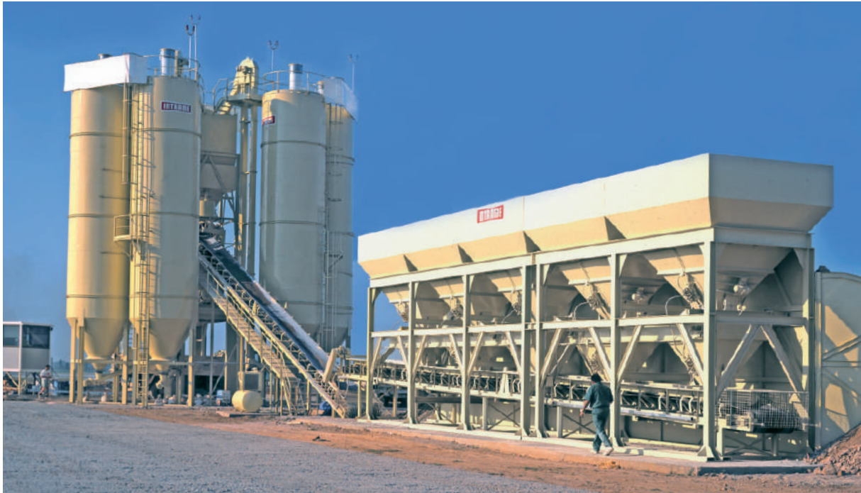
Concrete plant PH-150 equipped with a 3 m 3 twin shaft horizontal mixer working at Barcelona's airport.
