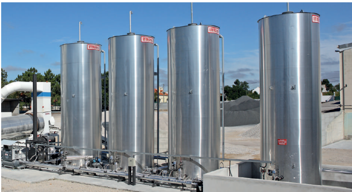
Vertical tanks heated by thermal oil.
