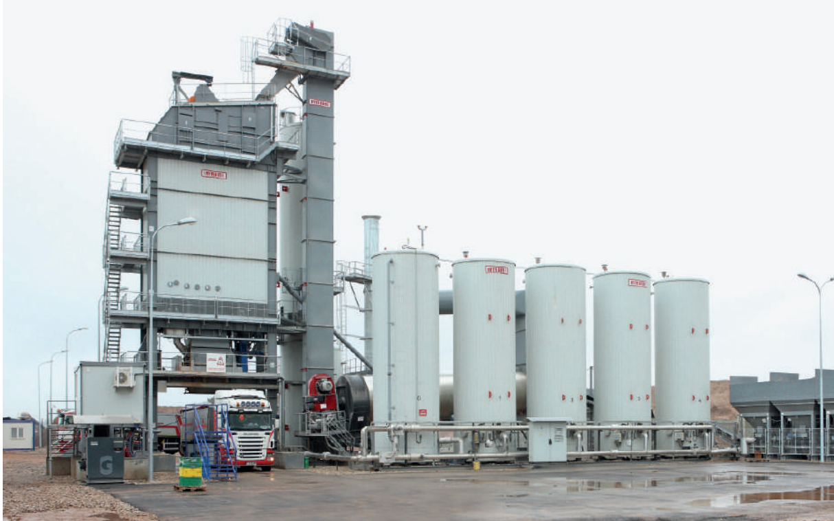
320 t/h asphalt plant (Poland). With InNOVA-G mixing tower. Equipped with 160 t capacity hot bins. Bitumen tanks electrically heated. Installed on metallic foundations. 4.500 kg mixer.
