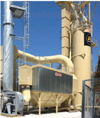
View of a bag house and a double silo for recovered dust and added filler in a RM-280.
